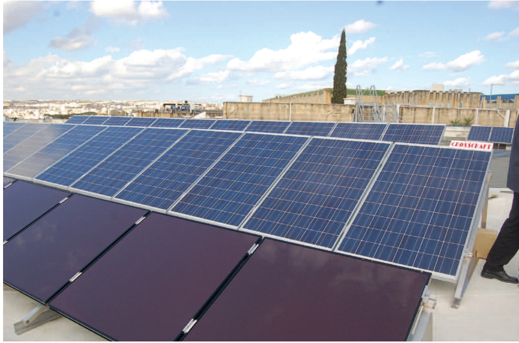
Abertax operates a series of solar panels from its office to help evaluate its battery management technology.
